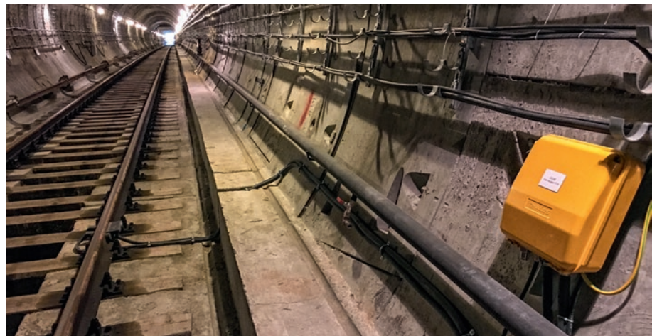
Wheel sensor Sk30K and EAK30K installed in Baku Metro tunnel
